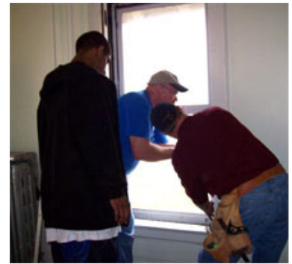
John Schlumbohm, David Hoffer and Ryan Martin work on the first window installation.
